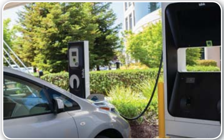
Evernote received grant funding to help defray the cost of its 10 Level 2 workplace chargers.
